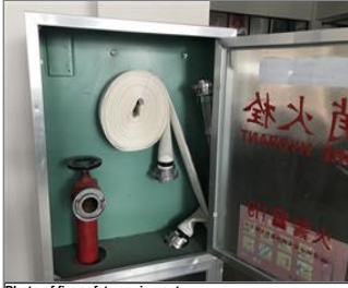
Photo of fire safety equipment 42 Fire hydrant.JPG
