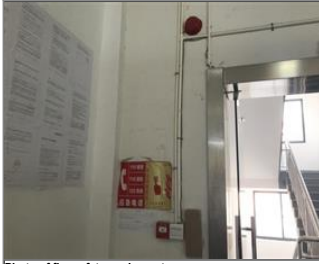
Photo of fire safety equipment 43 Fire alarm.JPG
