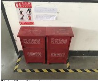
Photo of fire safety equipment 41 Fire extinguishers.JPG
